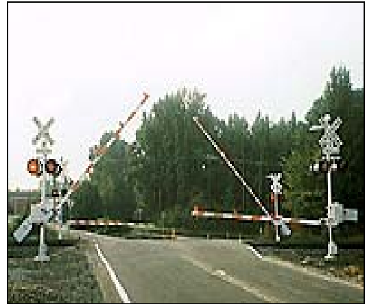
Figure 4 4-Quad Gates at West Craighead Road, Charlotte, NC
