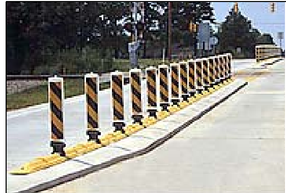
Figure 6 Traffic Channelization Device at Hickory Ridge Road, Harrisburg, NC
